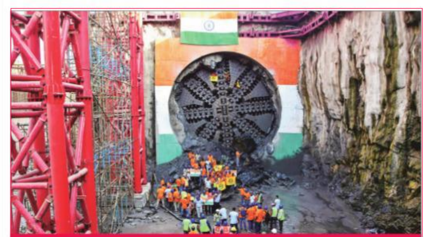
Workers and officials celebrate the breakthrough of the second tunnel from Swarajya Bhumi (Girgaon Chowpatty) to Priyadarshini Park of the Mumbai Coastal Road Project on Tuesday
